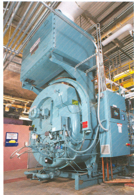
ROCKVILLE GENERAL HOSPITAL INSTALLED A NEW CLEAVER BROOKS FIRETUBE BOILER AND SAVED 15% IN FUEL COSTS AND REALIZED A 600,000 LB REDUCTION IN GREENHOUSE GASES.
